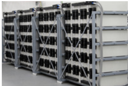
Energy Storage System
