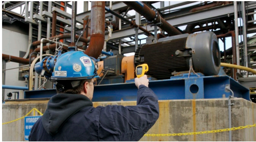
This is a 700 hp motor used to run the Equa-Chlor hydrogen compressor. Woelk has had typical readings around 75 °F to 80 °F. He is measuring the external surface of the motor, compressor, and gearbox.
