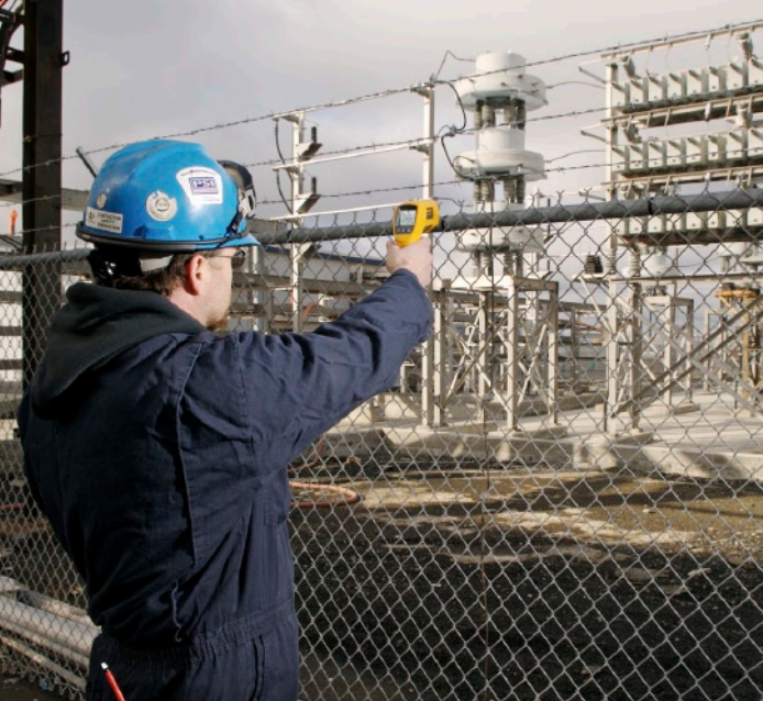
This is the plant's harmonic filter bank. Woelk is checking capacitors, insulators, and terminations. The temperatures of these connections varies with ambient air and plant load.
