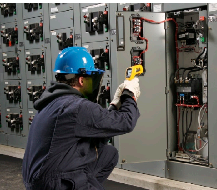
This is a motor starter bucket for a 60 hp motor. Woelk is checking fuses and terminations. He usually sees about 120 °F to 130 °F on components in the MCCs.
