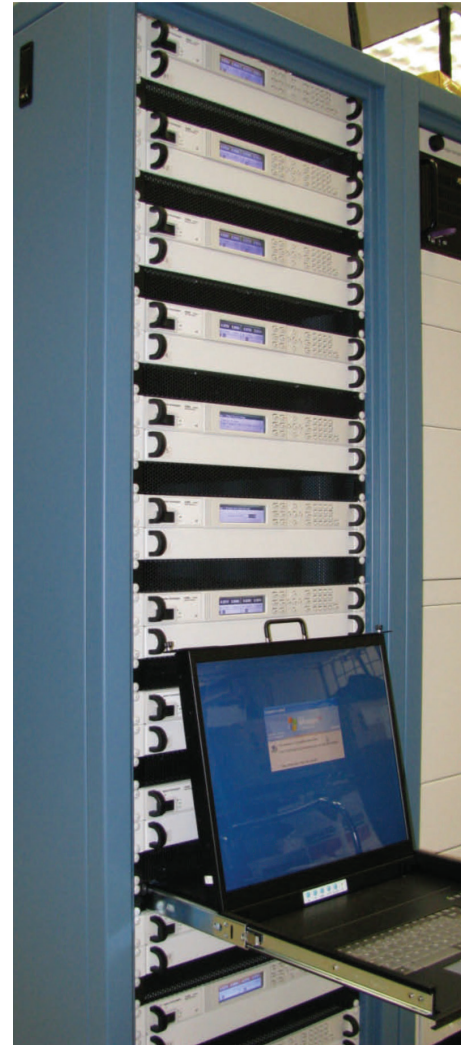
Figure 6. Custom turnkey system
