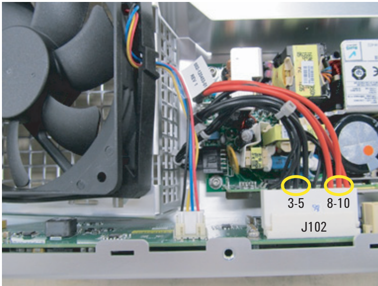
Figure 13 Verify power supply DC output
