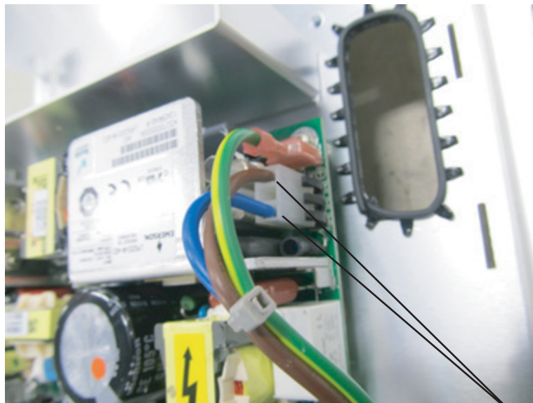
Verify AC potential between these two points
