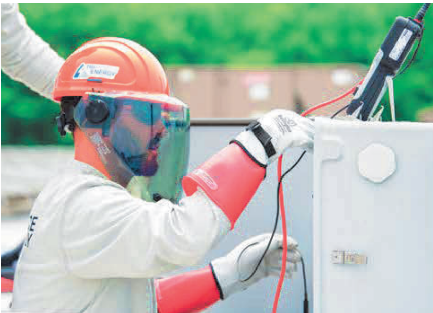
Figures 4-19 and 4-20: Technician wearing appropriate PPE while taking voltage measurements in a PV combiner box.
