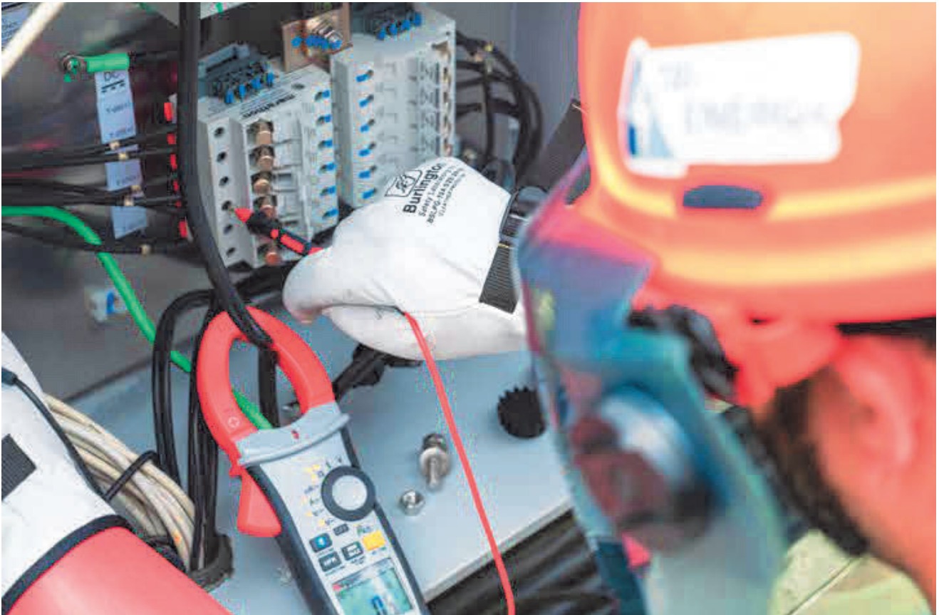
Figure 4-22: By applying the red lead (shown) and black lead (not shown) at different terminals in the PV combiner box, the technician can measure voltage down to the individual string level.
