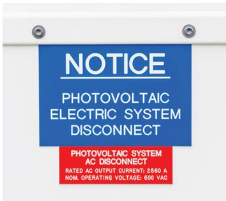
Figure 5-23: Current measurements should be verified at the PV system AC disconnect.
