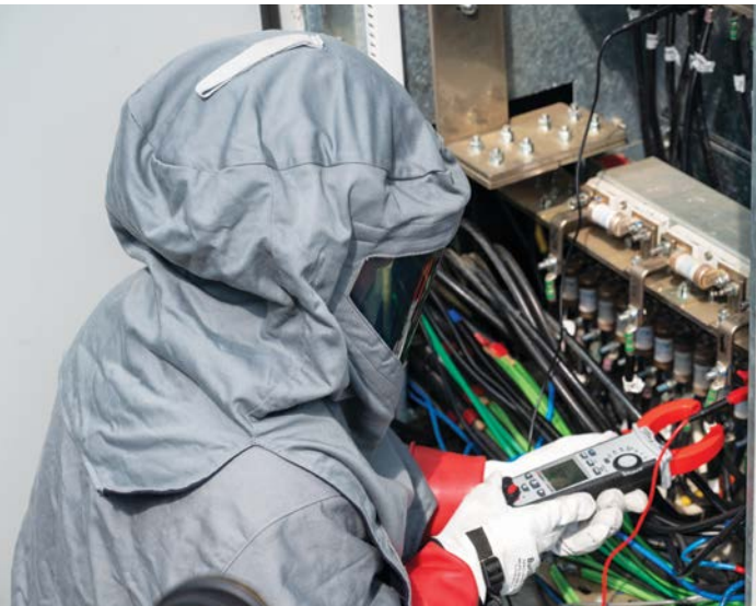
Figure 5-18: PV systems can operate at dangerously high amperages. Technicians should be aware of the risks associated with the expected system current and voltage, and should wear appropriate PPE.
