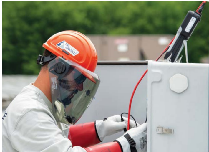
Figure 6-15: Technicians should understand the electrical hazards before they visit a site and should wear appropriate PPE.
