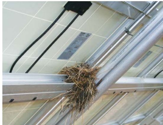
Figure 6-6: Animals nesting on and around PV system conductors can create damage, potentially causing ground faults.
